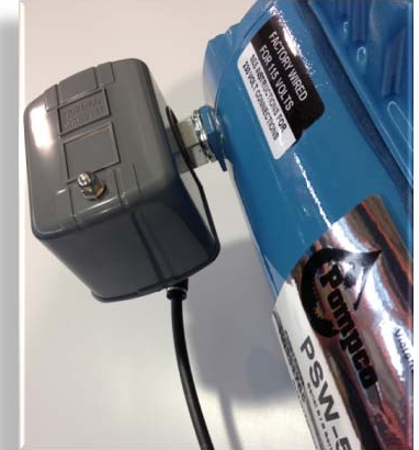
Figure 1: Pressure Switch Location
